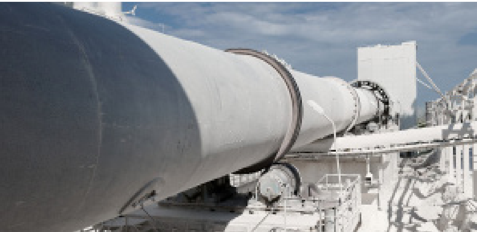
Calcium carbonate turning furnace with large pipe at cement plant.
